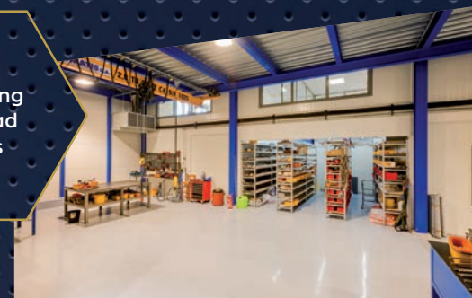
Single-girder underhung crane, 5 t x 15 m, with Verlinde lifting equipment. Client: Kotronic Packaging 2016, Efpalio, Phocis
