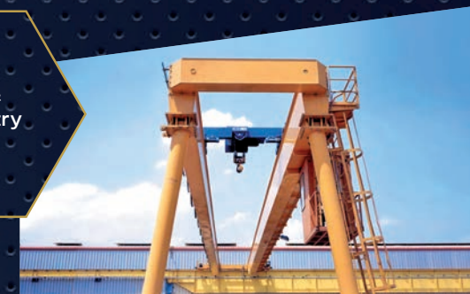
2 semi-gantry cranes, 10 t x 30 m, with Demag lifting equipment. Client: Corinth Pipeworks 2000, Thisvi Industrial Area, Boeotia
